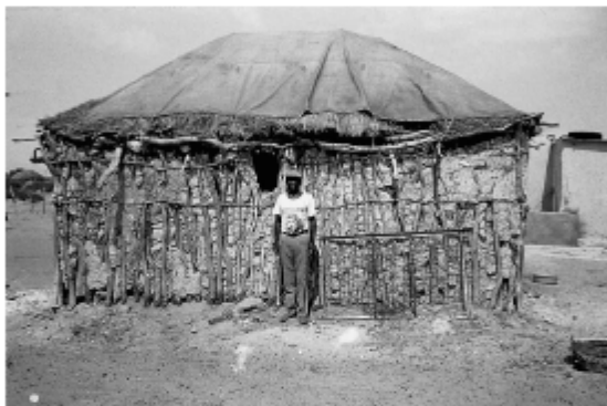
Fig. 3. Vertical poles with mud in-fill showing the damage caused by rainfall.
